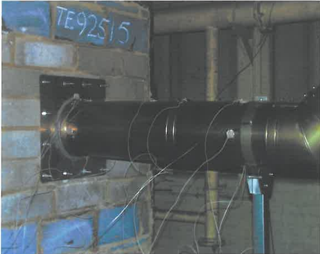
Plate 5 Chimney and penetration seal immediately after furnace shutdown at 246min
