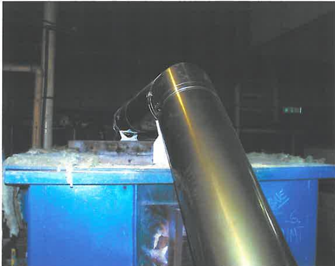
Plate 6 Showing typical condition of chimney system immediately after furnace shutdown at 246min
